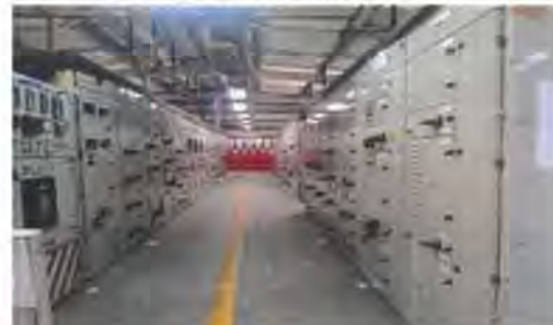
CS - 9 Electric Sub Station
