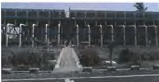
CS - 9 Gas After Cooler
