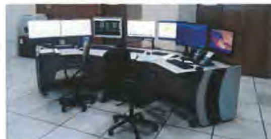
CS - 9 Local Control Room
