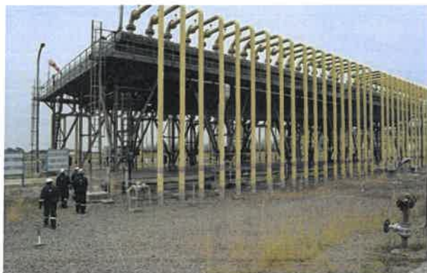
CS - 1 Gas After Cooler
