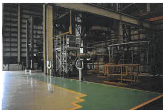
CS - 1 Compressor Station
